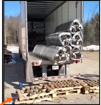
Below—3 RP4XL Roll Pullers Pulling a 75 Roll Tier Of Paving Fabric in 25 Banded Groups of 3 Rolls in one pull. I WAS AMAZED. Photos by contractor choosing to remain anonymous
